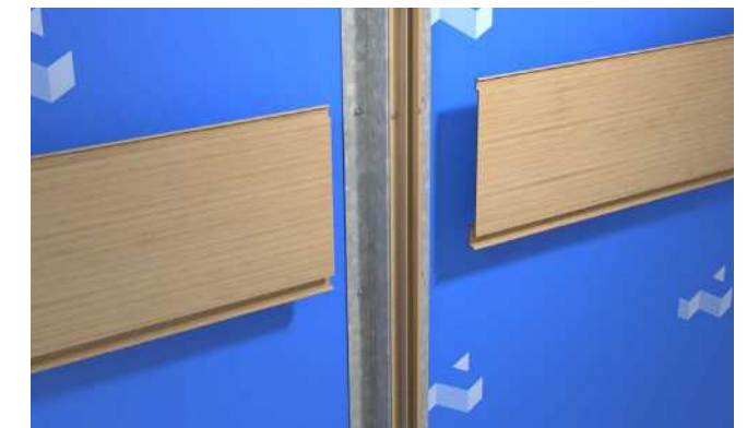
Step 2. Place cladding board on either side of the Female Joiner Trim and secure boards with screws.
